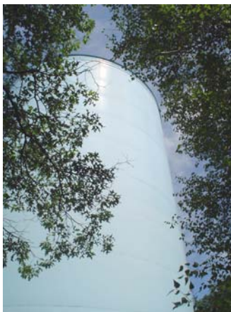
One million gallon tank
